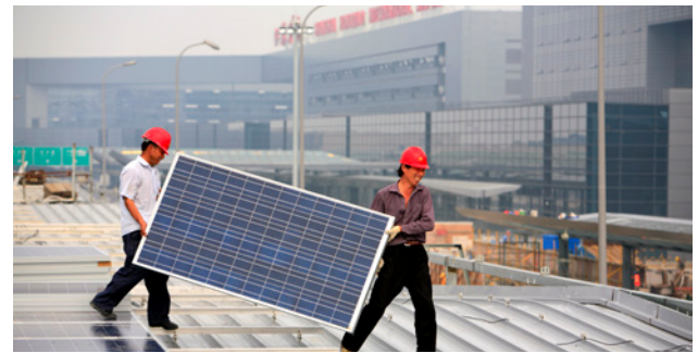
Installation of solar photovoltaic panels on the roof of the Hongqiao Railway Station in Shanghai
